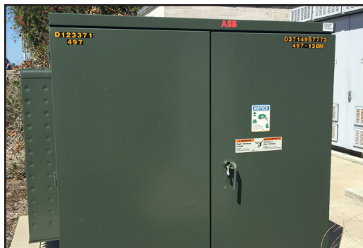
SDG&amp;E Padmount Transformer
