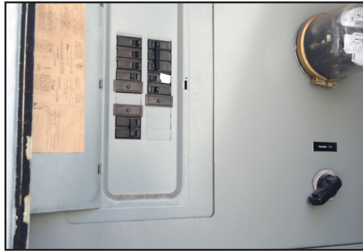
Main Distribution Board with Interior Panel Board
