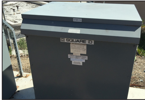
480-120/208V Transformer serving building 2300
