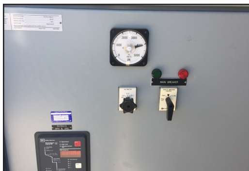
Main 5kV Breaker Cubicle and Protection
