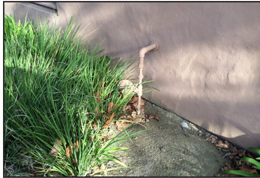
Building 400 - Gas supply into building with gas pressure regulator along building exterior.
