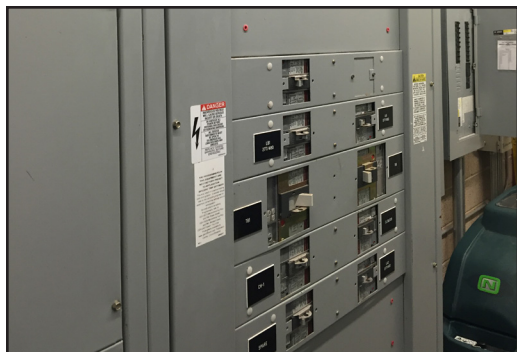
Main Distribution Board
