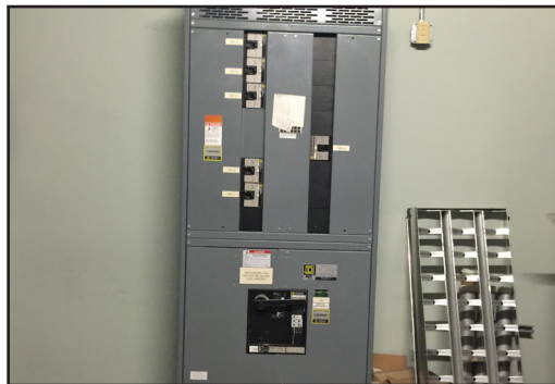
Main Distribution Board
