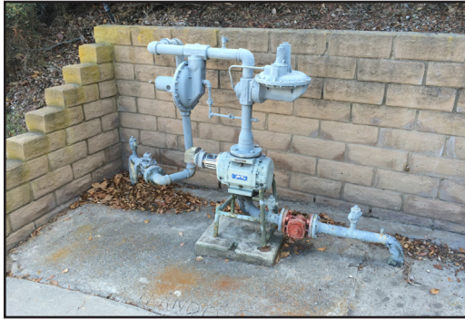
SDG&E gas meter along Barnard Drive.
