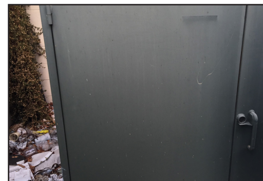
4.16kV-120/208V Padmount transformer
