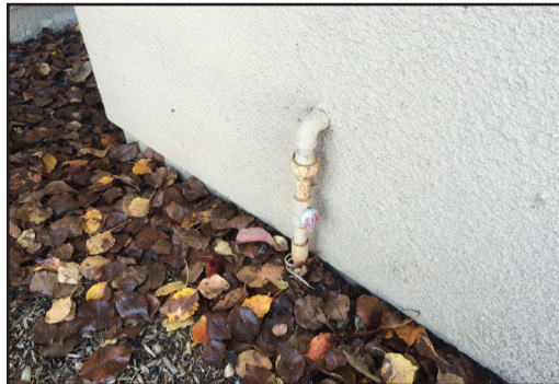
Building 4400 - Low pressure gas into building at north-west corner.
