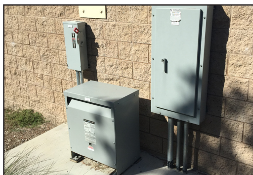
480-120/208V Transformer and 120/208V Panel Board
