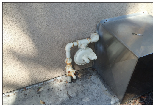
Building 4500 - Above grade gas pressure regulator along building exterior.
