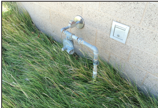
Building 2200 - Above grade gas pressure regulator along building exterior.
