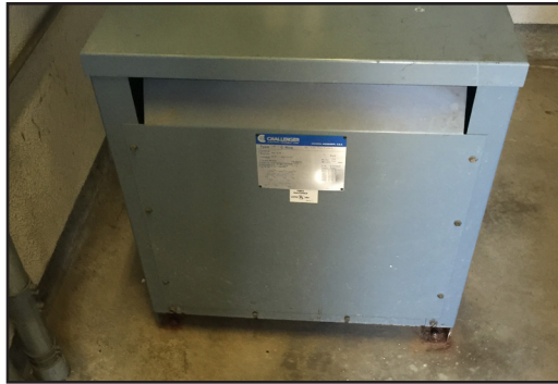
Building 900 - Typical 480-120/208V transformer
