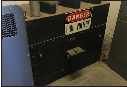
5kV Oil Fused Cutout
