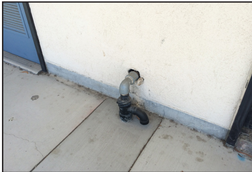
Building 3500 - Low pressure gas into building.
