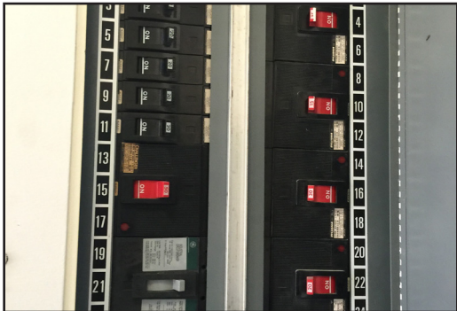
Building 600 - Typical panelboard
