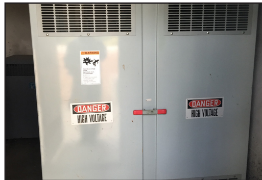
4.16kV-277/480V Dry-type Transformer
