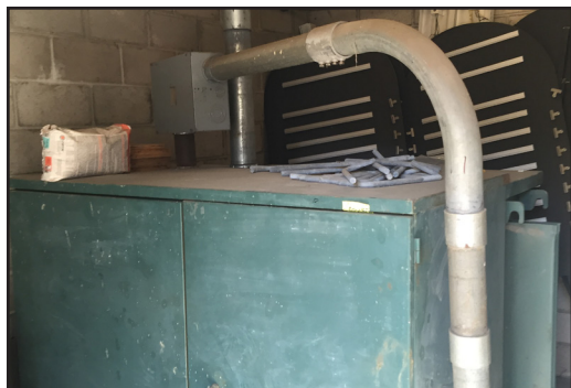
Main 4.16kV-120/208V Transformer
