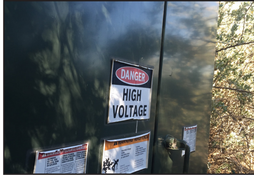
Liquid Filled Padmount Transformer
