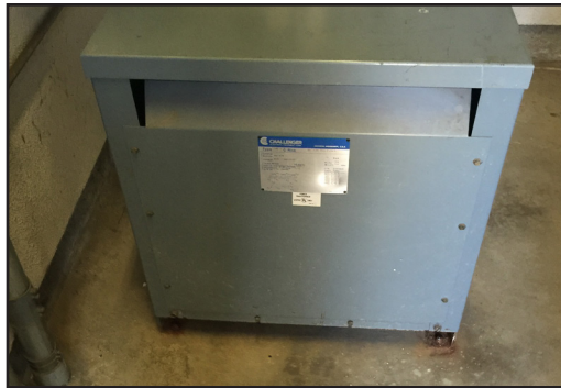
Typical 480-120/208V transformer
