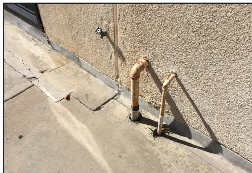
Building 3000 - Low pressure gas into building.
