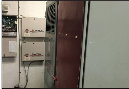
Main 4.16kV-277/480V Dry-type Transformer
