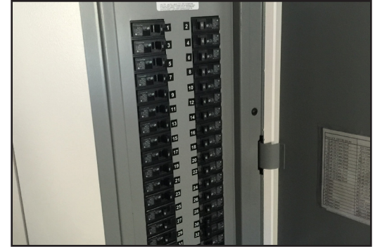
Building 1000 - 120/208V panelboard
