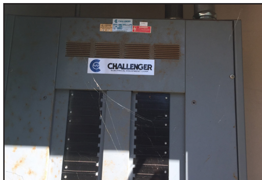
Building 100 - Main Distribution board
