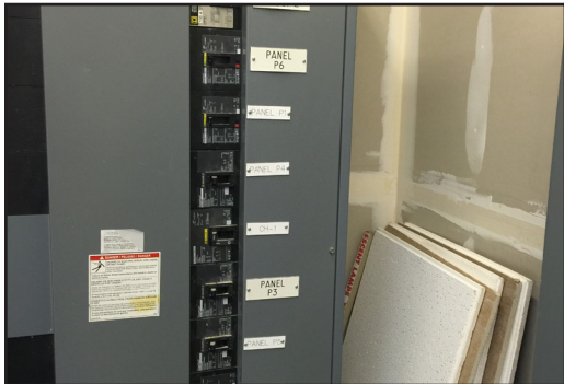
Main 2000A 120/208V Distribution Board
