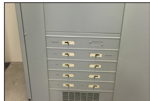
Main Distribution Board 277/480
