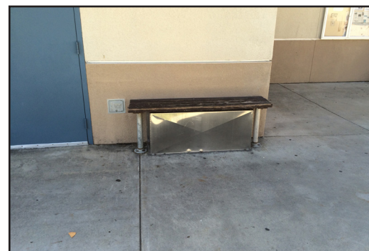
Building 4600 - Enclosure along the building exterior believed to house the gas pressure regulator with shut-off.
