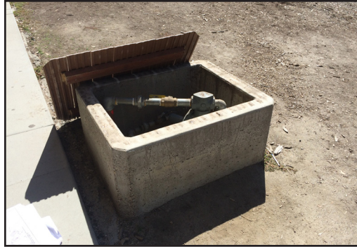
Building 3500 - Gas Pressure regulator inside concrete vault.
