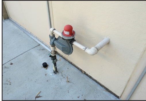
Building 2300 - Above grade gas pressure regulator along building exterior.
