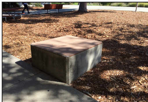
Building 4800 - Gas Pressure regulator inside concrete vault.
