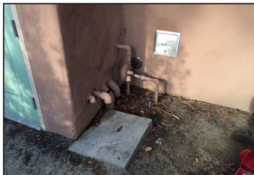
Building 200 - Gas supply into building with gas pressure regulator along building exterior.
