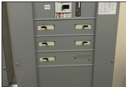
Main Distribution Board 120/208
