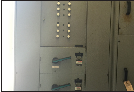
Building 600 - Main distribution board
