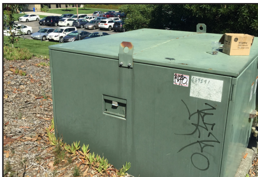
15kV Selector Switch
