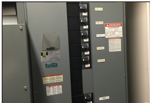
Main 120/208V Switchboard
