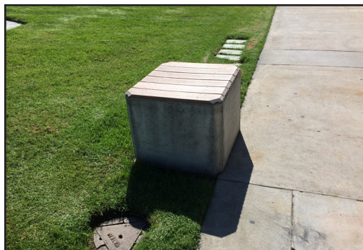
Building 3100 - Gas Pressure regulator inside concrete vault.
