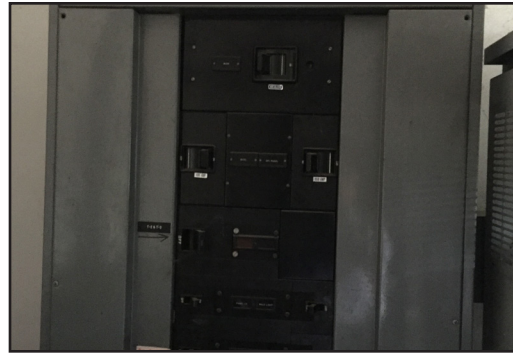
Main 277/480V Switchboard
