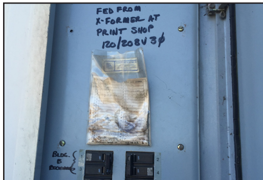
Main 120/208V Panel Board in T600
