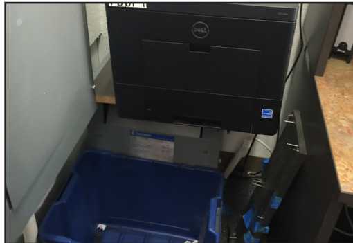
Building 700 - 480-120/208V transformer
