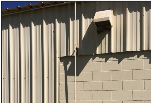
Building 5100 - Low pressure gas into building.
