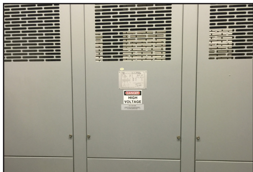
300kVA 4160-277/480V Dry-type Transformer
