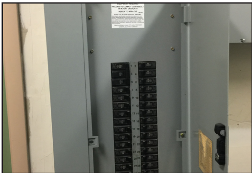
Building 900 - Typical panelboard
