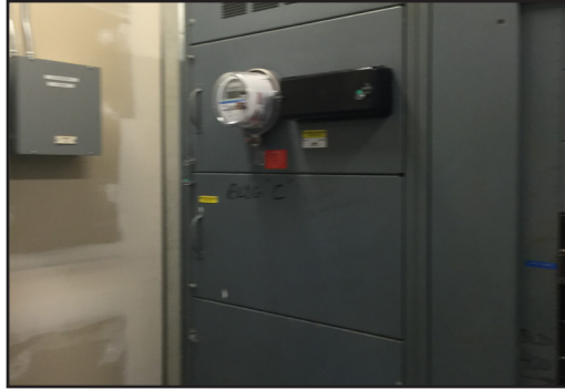
Typical Main distribution board with SDG&E meter
