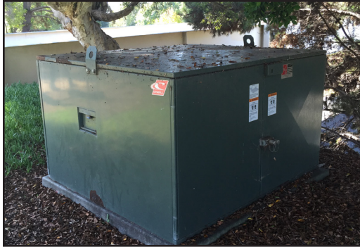
15kV Selector Switch
