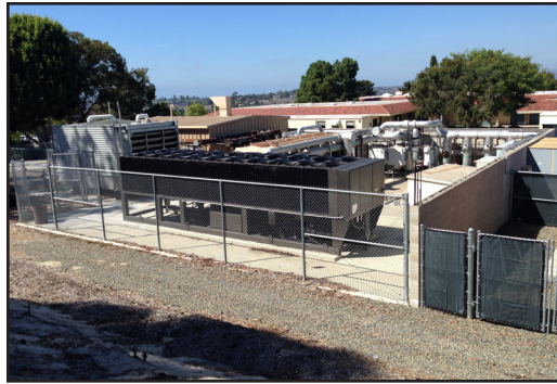
Central Plant Overview
