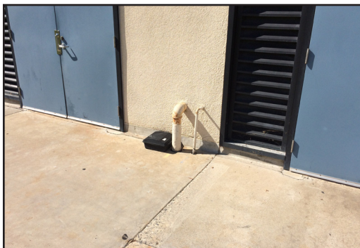
Building 3100 - Low pressure gas into building.
