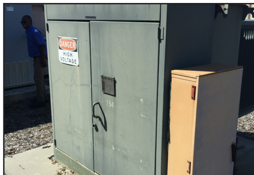
Abandoned Padmount Transformer
