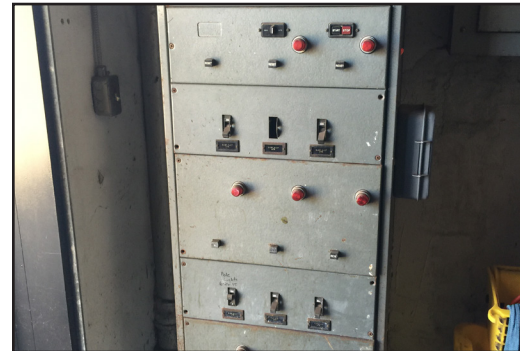
Motor Control Center
