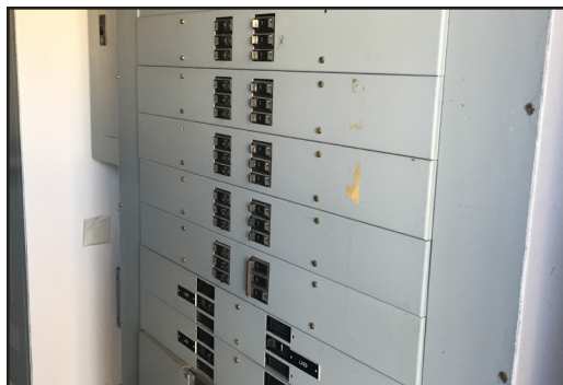
Main 1600A 120/208V Switchboard
