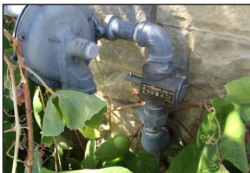
Building 1200 - Low pressure gas into building.
