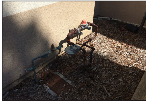
Building 4400 - Above grade gas pressure regulator along building exterior on the south side of the bldg.
