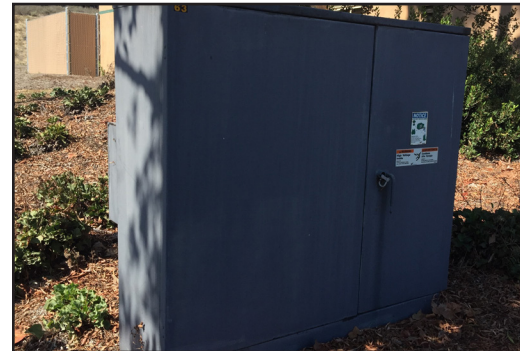
Building 700 - SDG&E pad mount transformer
