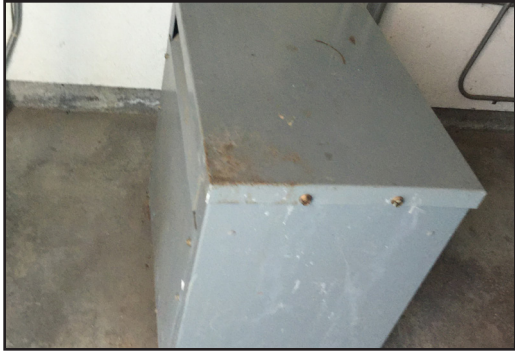
Building 600 - Typical panelboard
