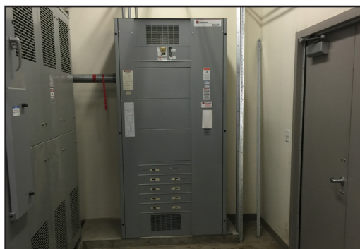
Main Equipment Room
