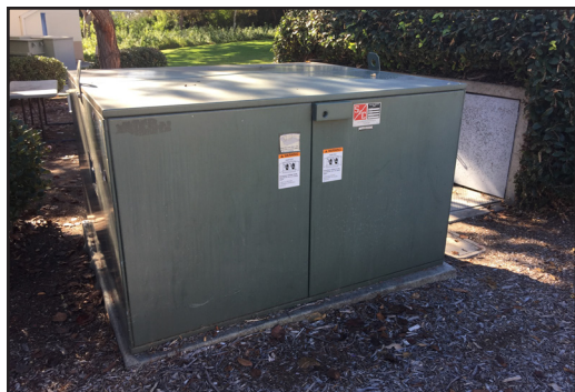
15kV Selector Switch
