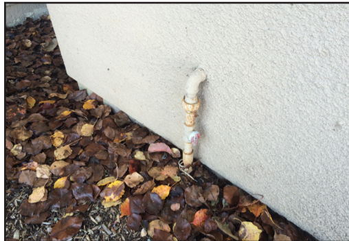
Building 7000 - Above grade gas pressure regulator along building exterior.
