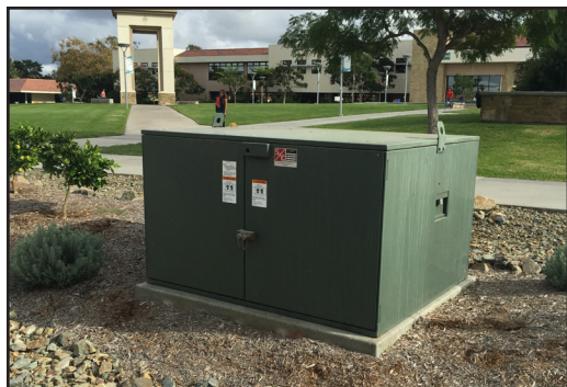
15kV Selector Switch
