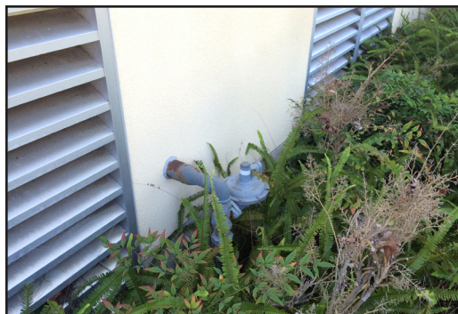
Building 8000 - Gas Pressure regulator inside underground vault.
