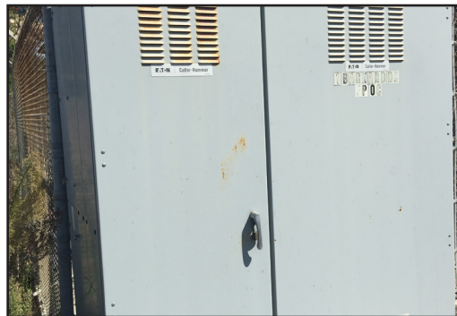
Main Distribution Board serving Fire Pump
