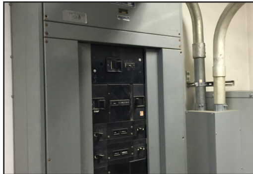
Main 800A 277/480V Switchboard
