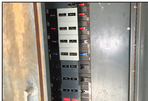
Main Distribution Board
