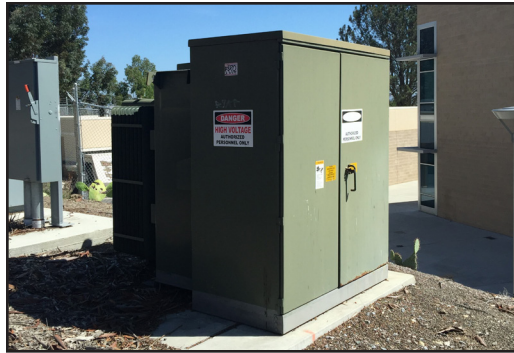
750kVA 4.16kV-277/480V Padmount Transformer
