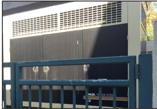
Generator Serving Existing Data Center
