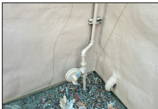
Building 200 - Gas supply into building with gas pressure regulator along building exterior.
