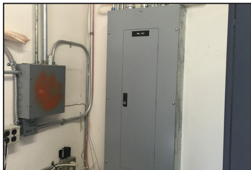
Building 100 - Panel boards Typ.
