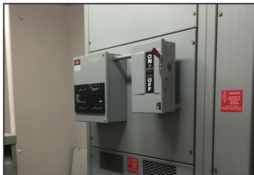
Main 1600A 120/208V Switchboard
