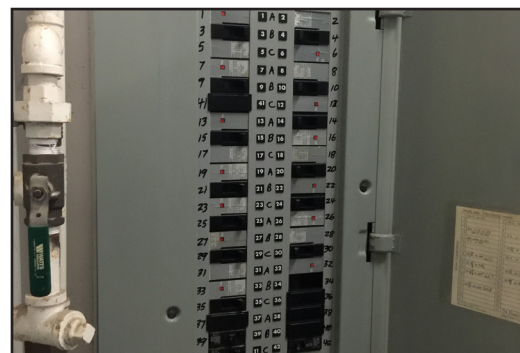
Building 500 - Typical panelboard
