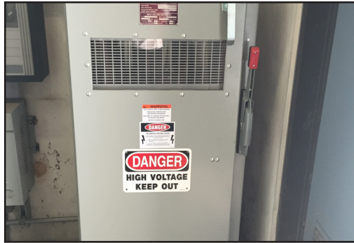
Main 5kV Switch
