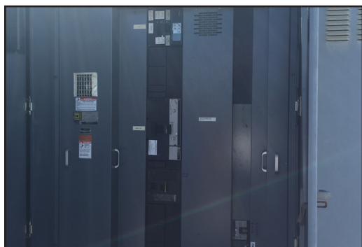
Main Distribution Board
