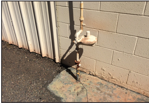
Building 5100 - Gas Pressure regulator inside underground vault.
