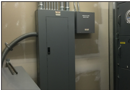
Building 900 - Typical panelboard
