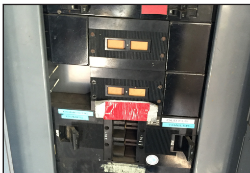
Main Distribution Board in Electrical Power House
