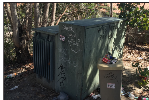
4.16kV-277/480V Padmount Transformer
