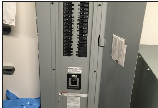
Building 1000 - 277/480V panelboard
