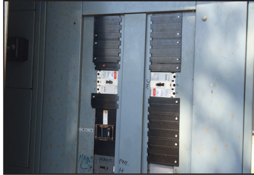
Building 700 - Main distribution board with SDG&E meter
