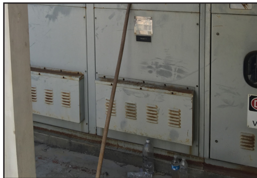
Main 277/480V Switchboard
