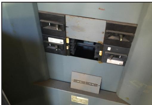
Main Distribution Board
