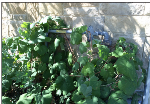
Building 1200 - Above grade gas pressure regulator along building exterior.
