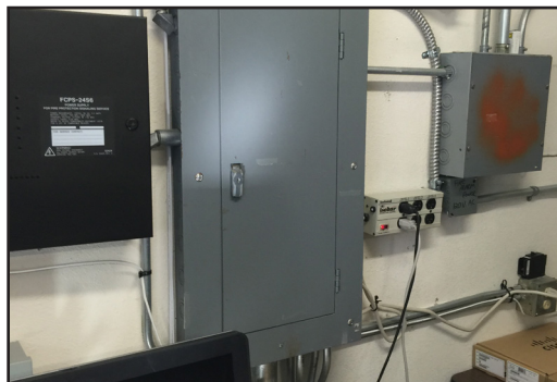
Building 100 - Panel boards Typical
