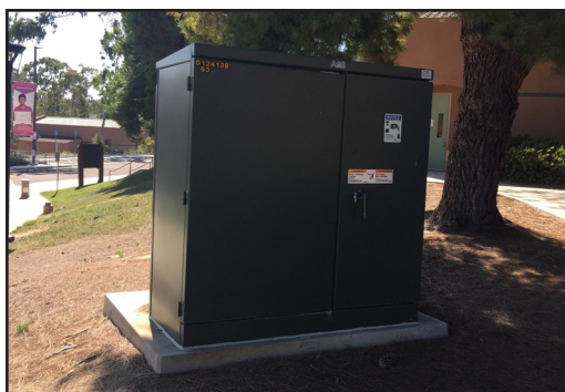
Building 500 - SDG&E pad mount transformer
