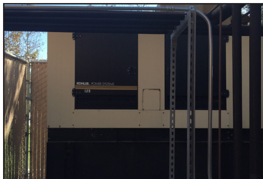
Building 100 - Generator for Data Center
