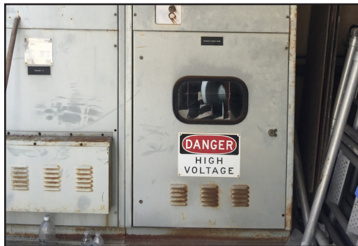
Main 5kV Switch
